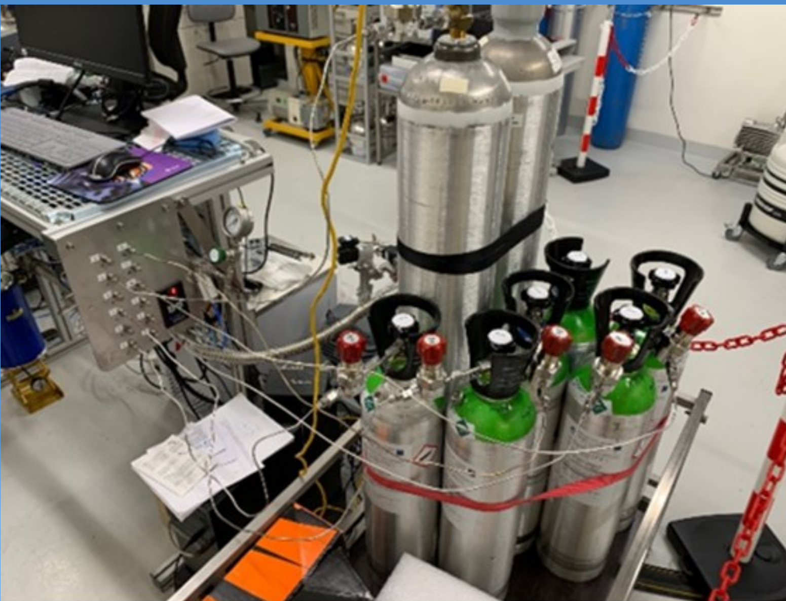
Photos of new sample cylinder inlet system (left) and close-up on new manual valve and pressure gauge
