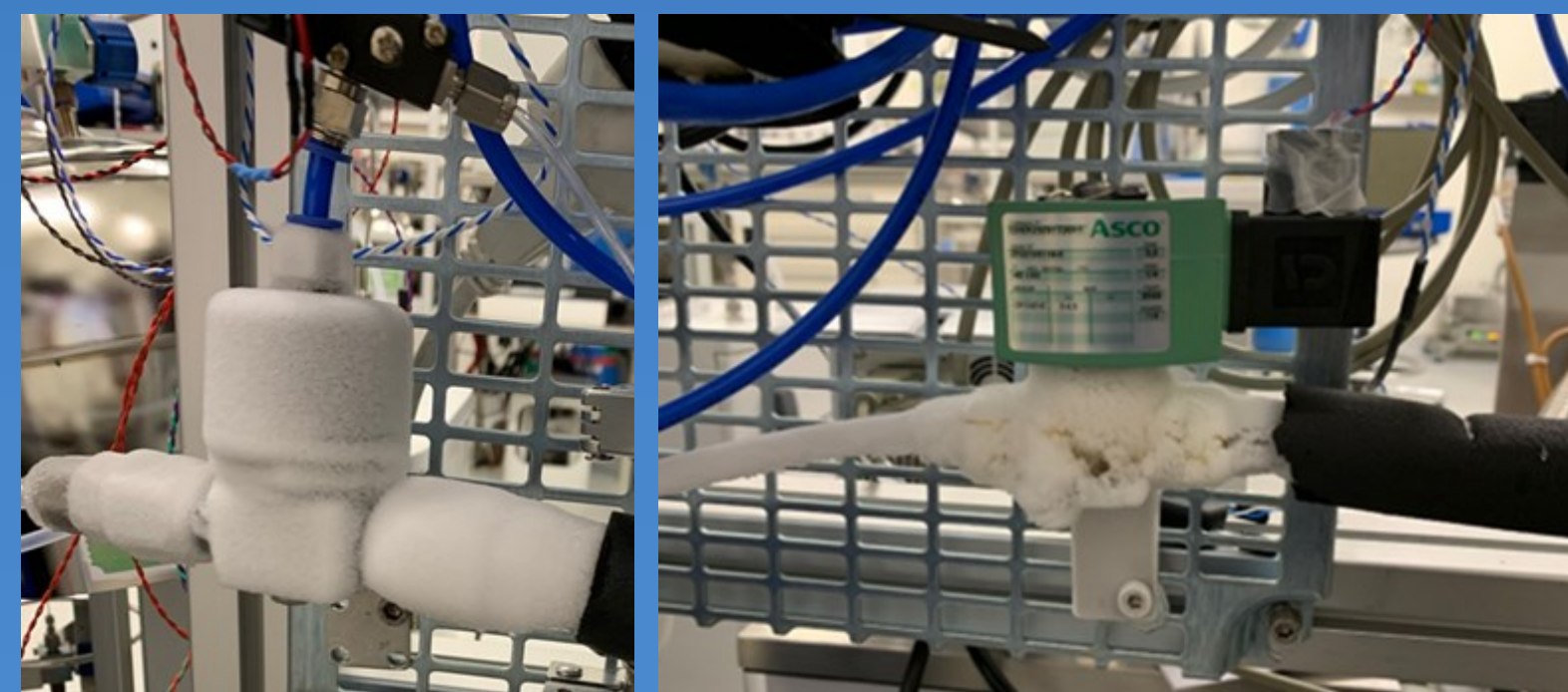
Photos of the valves used for controlling the cooling of all cold traps. Left is the old model and on the right the new one.
